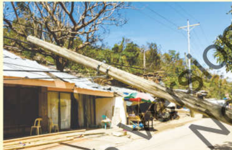
Infrastructure Damage by Earthquake
